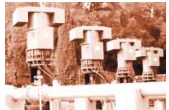
Medium voltage water pumps
