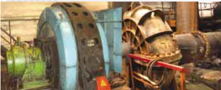
Synchronous motor driving an iron ore pump
