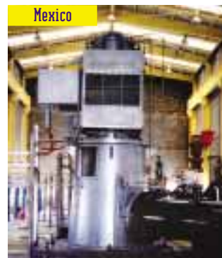
Mexico Four City Municipality Water Pumps at 4160V / 400A elevating Fresh water to 1800 Meters
