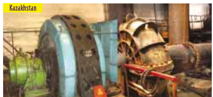
Kazakhstan Iron Ore Mud Pumps at 6000V / 500A (Synchronous Motors)
