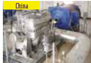
China Liquid Gas Booster Compressor 6600V / 600A
