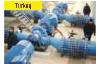
Turkey Three City Municipality Fresh Water Pumps 3300V / 300A
